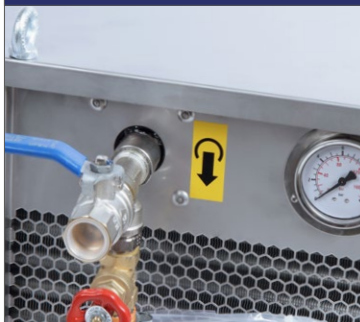
Coolant recirculation and pressure gauge
