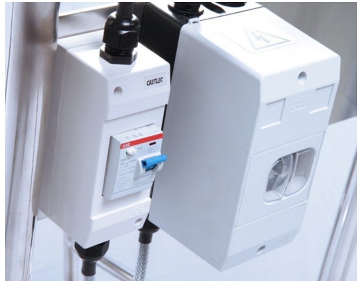
Power supply and RCD
